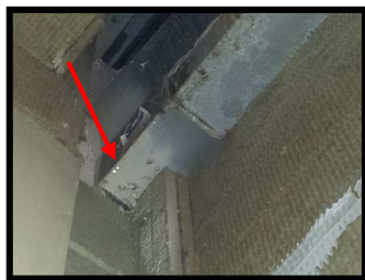
Water leaking into stockroom below
