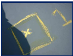
Small breaches found on the roof
