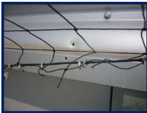
Some of the many missing fixings where water penetration occurs
